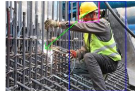
(c) failed to identify the welding area
