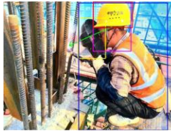
(b) welding area is obscured
